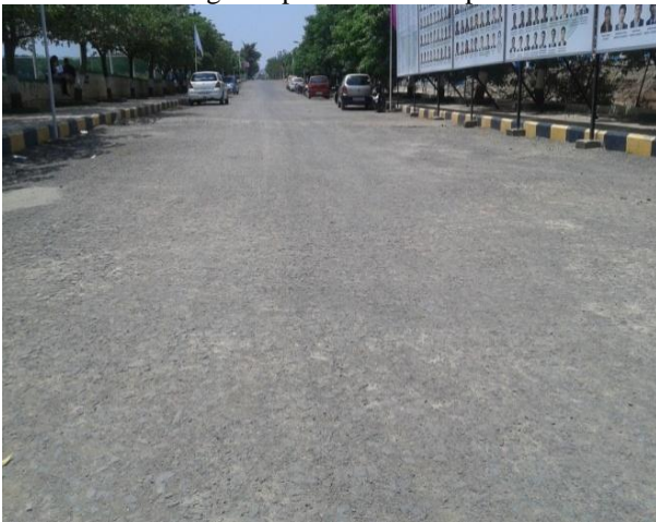
Fig.2 Rough road Condition
