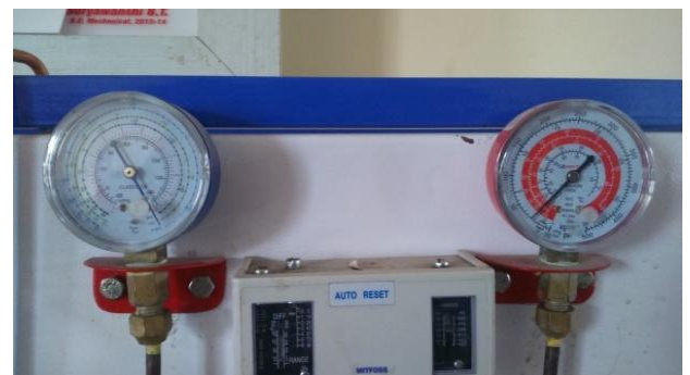
Fig.7 HP & LP Gauges
