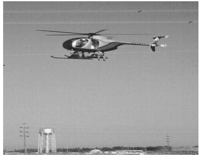
Figure2: A helicopter flying along an electric transmission line, with a lineman
